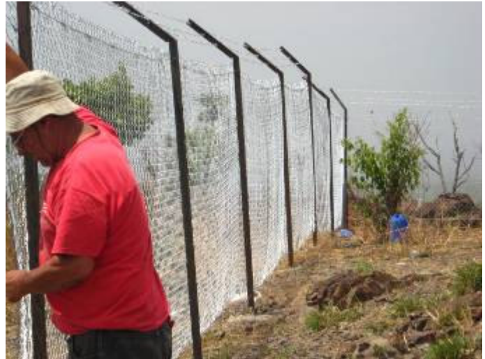
Figure 6 Engineer David Firth working on the fence project on top of Gordon Mt
